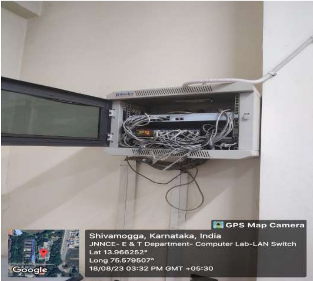
ETE DEPARTMENT: NETWORK SWITCH
